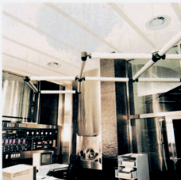
Control room: König Brewery, Duisburg
