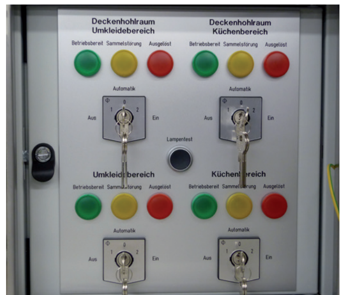
Fire brigade indicator panel FBIP
