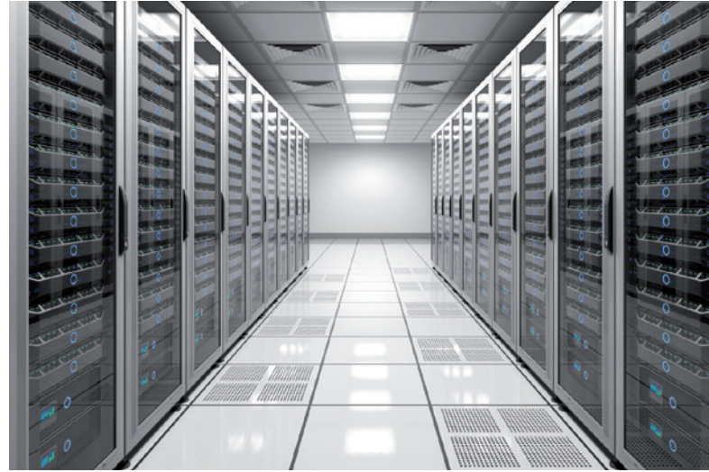
Example of a server room
